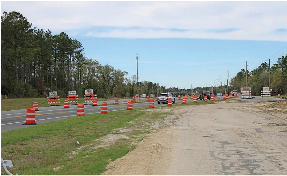
DOT officials acknowledged that the $25 million expansion of U.S. Highway 319 is behind schedule and won't be finished on time.
